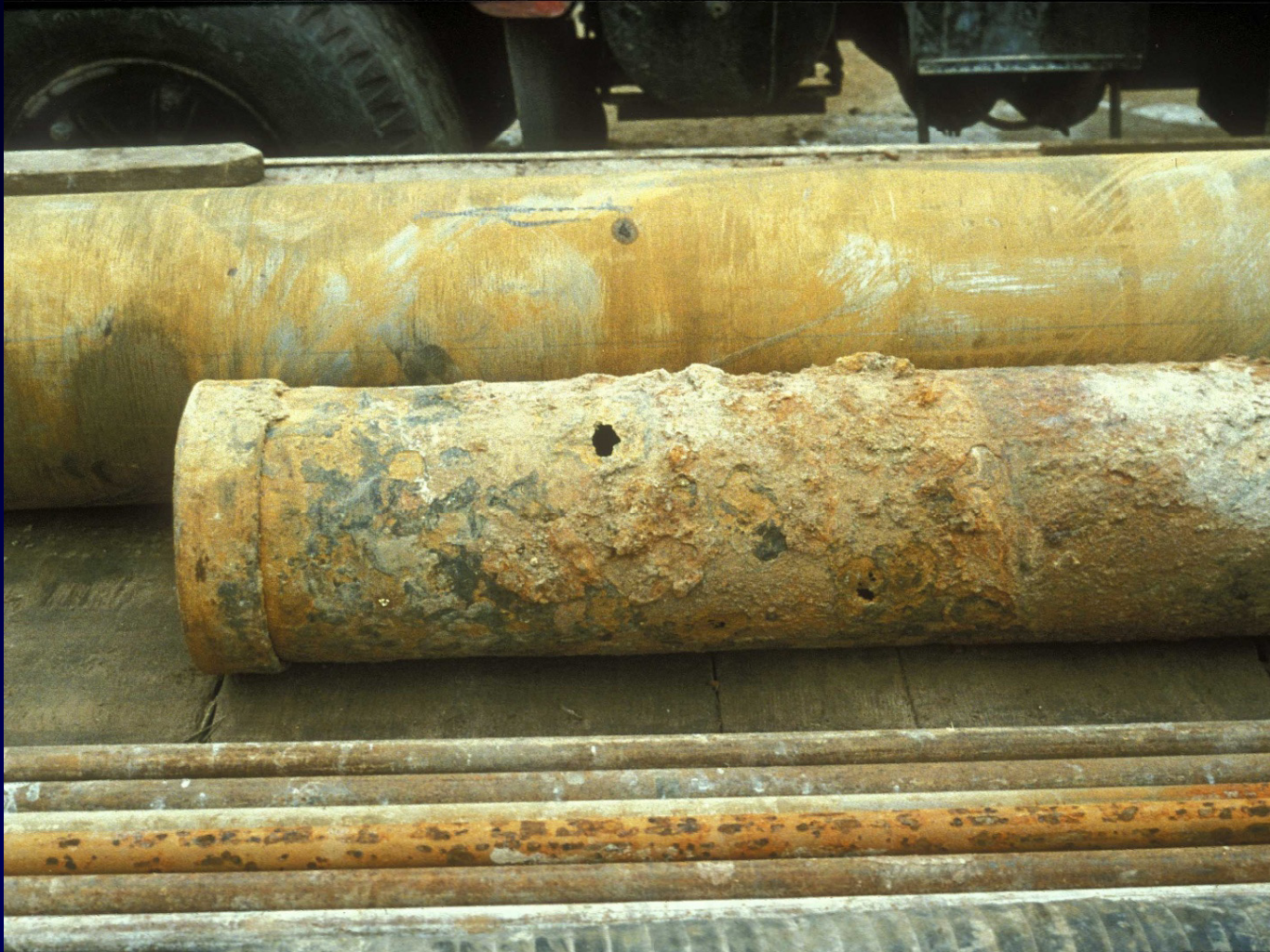
Well casing, Benton, Wisconsin
